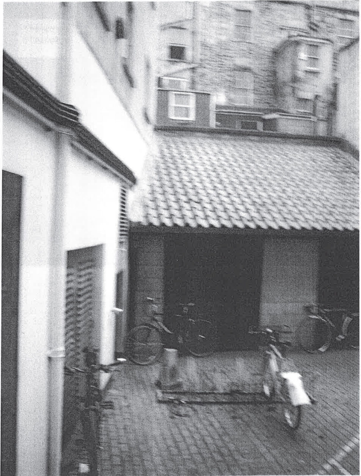
Photo3: showing height of drop from perimeter wall to IPL courtyard and access to internal areas of the premises
